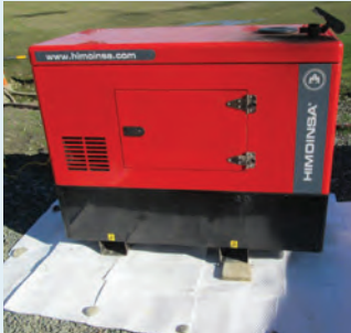
A generator with spill protection in place on a work site.
