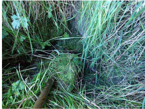
Figure ii. Evidence of underground tunnelling by rainfall in the northern gully.
