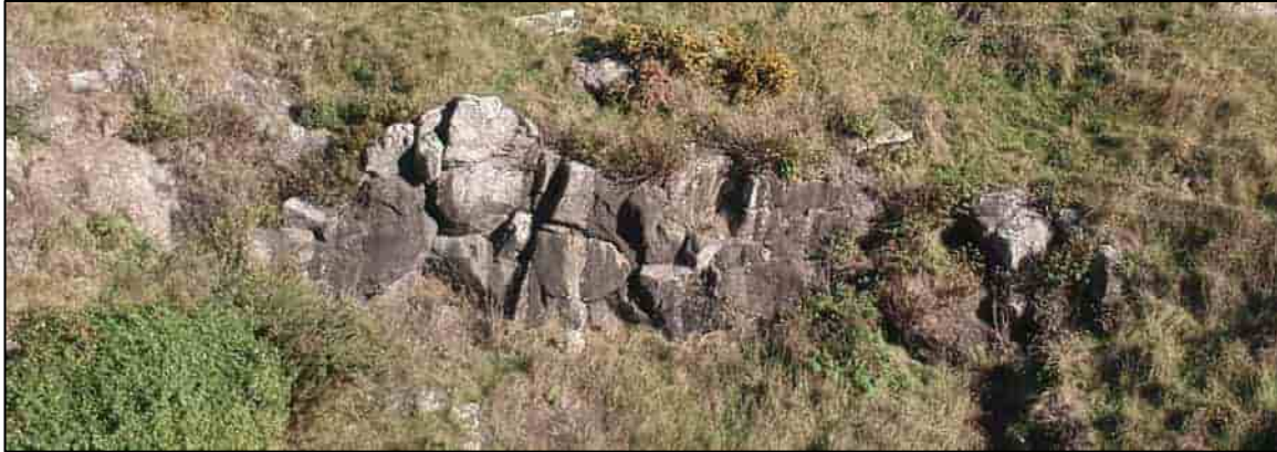
Photo 3: View of jointed basalt and what appears to be loose blocks in an outcrop source area.
