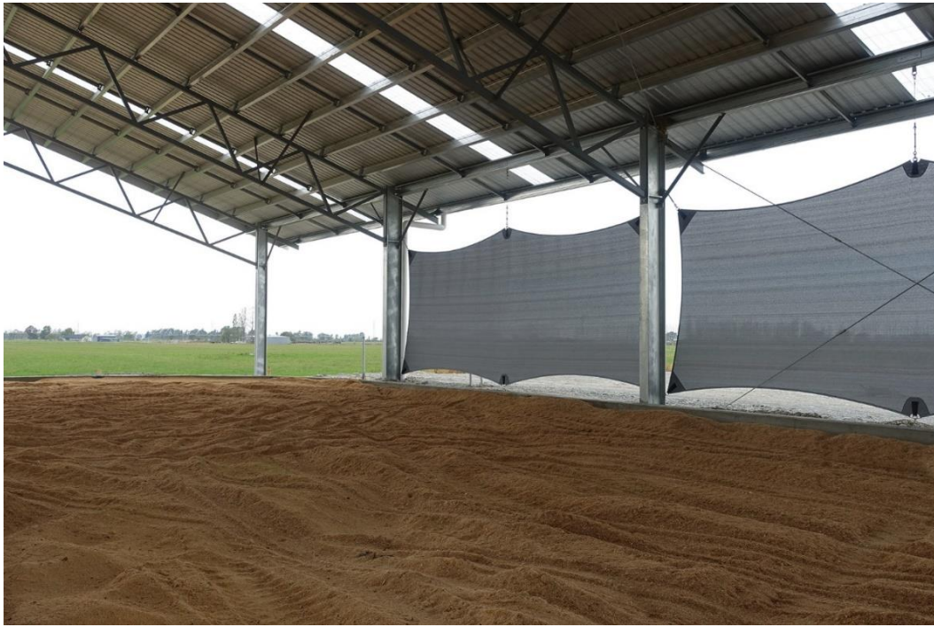
Photo 15. Shade sails used to reduce wind and rain on exposed sides.
