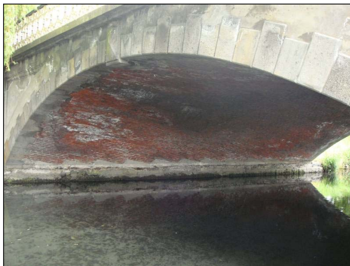
Figure 1.18. Brick arch on concrete foundations with basalt stone voussoirs on the arch.
