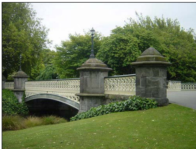
Figure 1.16. Elaborate cast iron balustrade of the earlier Victoria Bridge and stone abutments and posts. Source: www.flickr.com
