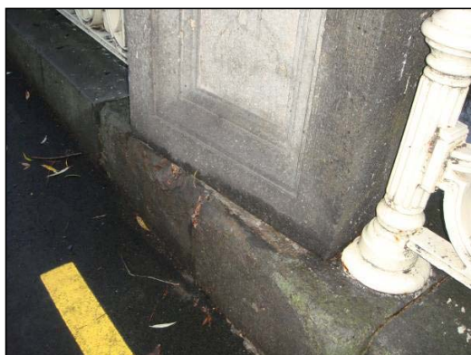
Figure 1.21. Rotation of pillar on bridge. Source: DPAL, 2012
