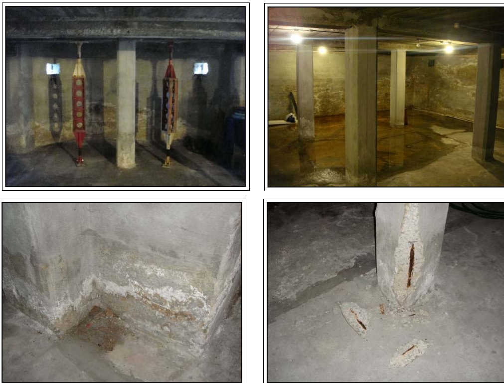
Figures 1.75.- 1.78. (Top left) Steel props in basement, 2012; (Top right) water in basement, 2012. Lower left) signs of efflorescence on wall, 2012; (Lower right) rising damp in columns, 2012. Source: DPAL
