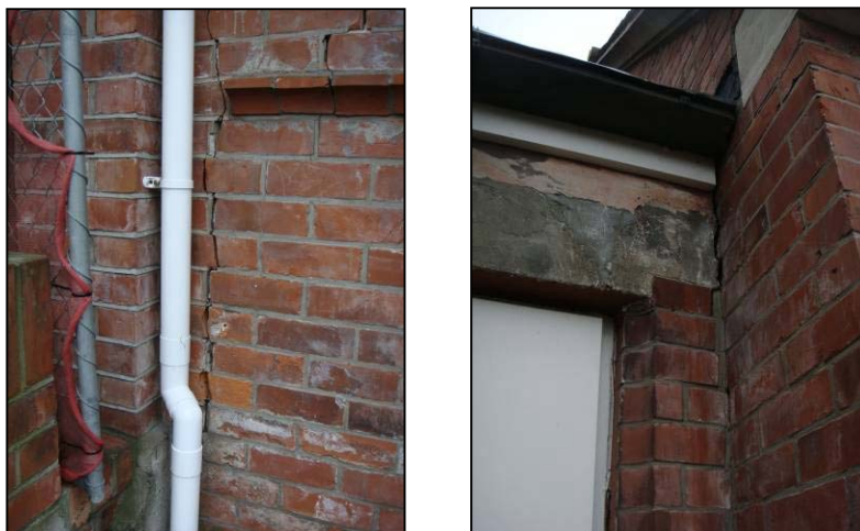
Figure 1.79. Cracks in exterior brickwork of Chapel, 2012. Source: DPAL
