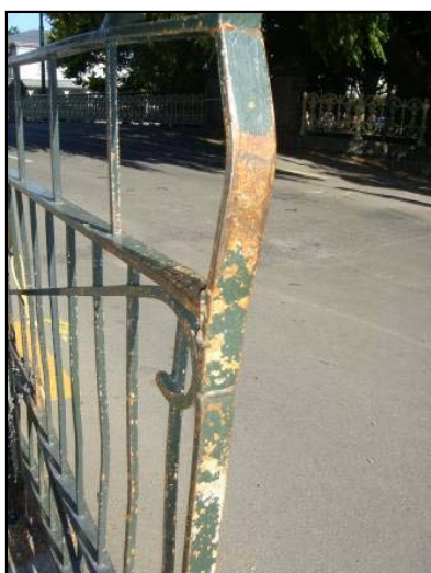
Figure 1.37. Buckled and rusting gate with chipped paint. Source: DPAL,2012
