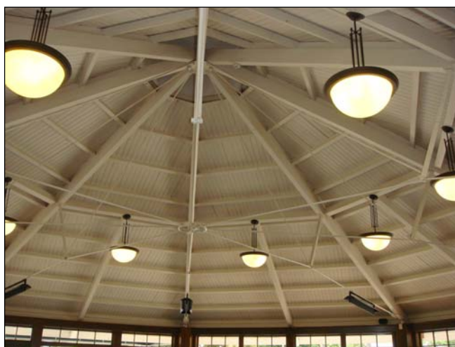
Figure 1.89. Octagonal timber ceiling with timber rafters splayed to each corner supporting the roof.
