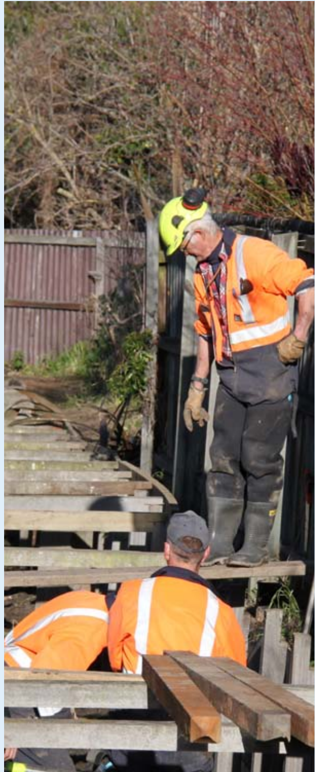
City Care staff carry out repairs to earthquake-damaged waterways as part of Christchurch's infrastructure rebuild.
